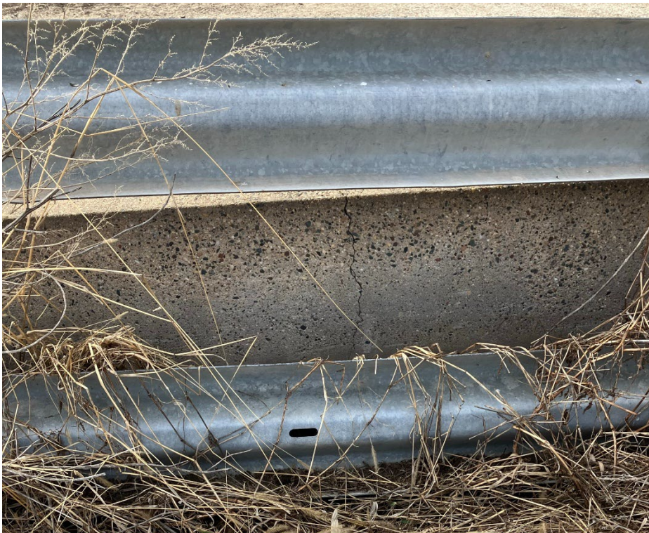
Once of several cracks in silage bunker walls
